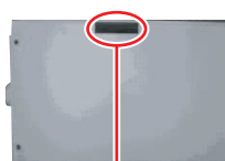
Gap on the side
